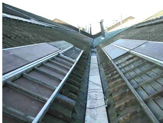
Figure 6 A partially boarded out valley gutter (another line of boards needed to reach 2 nd purlin line)
